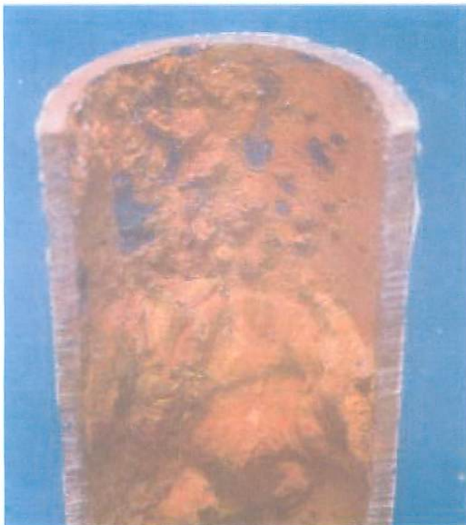
Galvanized pipe heavily corroded
