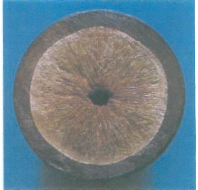
Galvanized pipe heavily scaled
