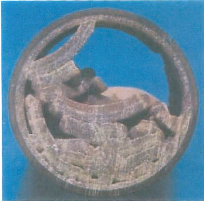
Copper pipe with scale plug
